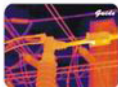
Inspect electricity hot point
