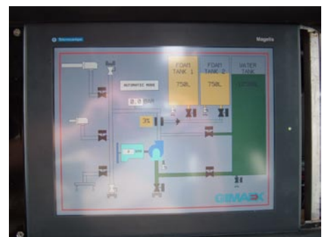
Display for the hydraulic circuit
